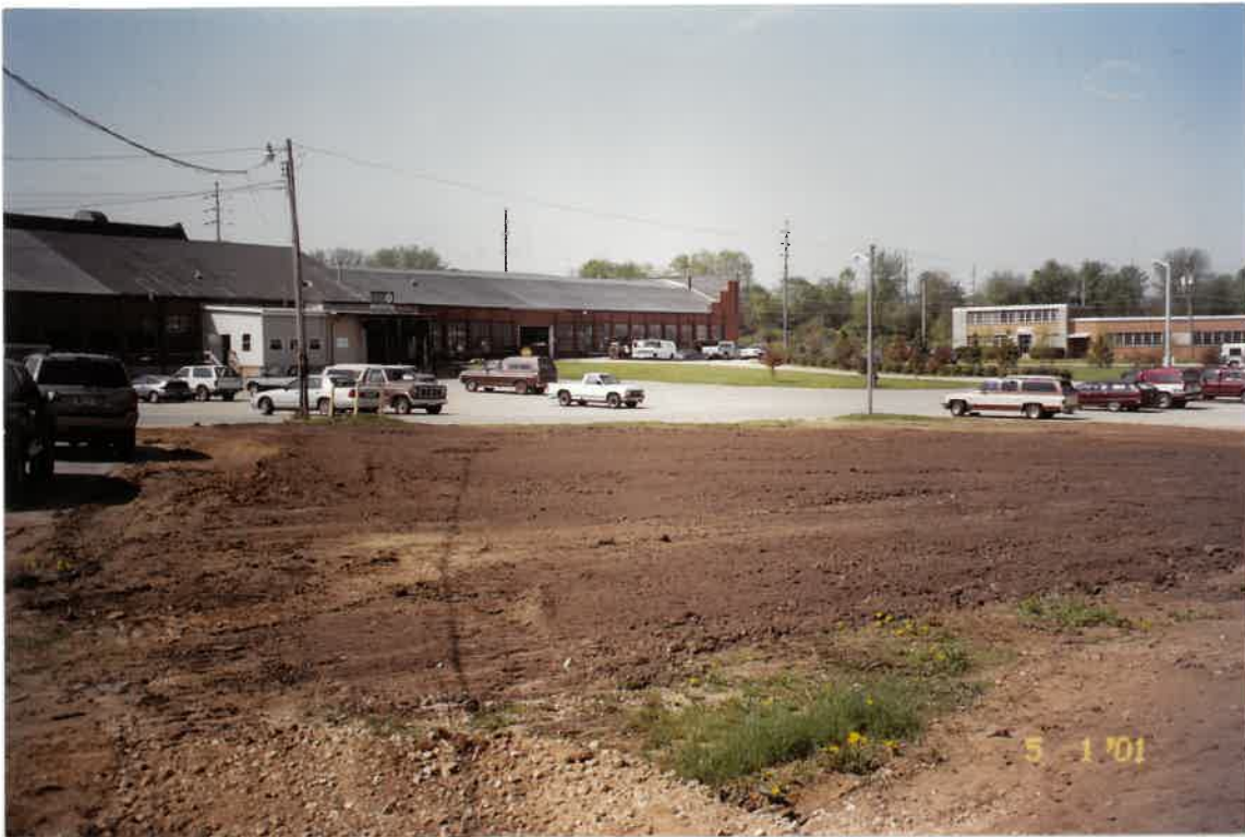
Photograph 11 May 1, 2001 Description: Restoration work partially completed for Cyanide Vault and Lagoon No. 0 (Topsoil placed and fine graded).
