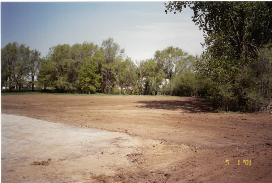
Photograph 12 May 1, 2001 Description: Restoration work in progress on Lagoon No. 1A (Topsoil placed and fine graded).
