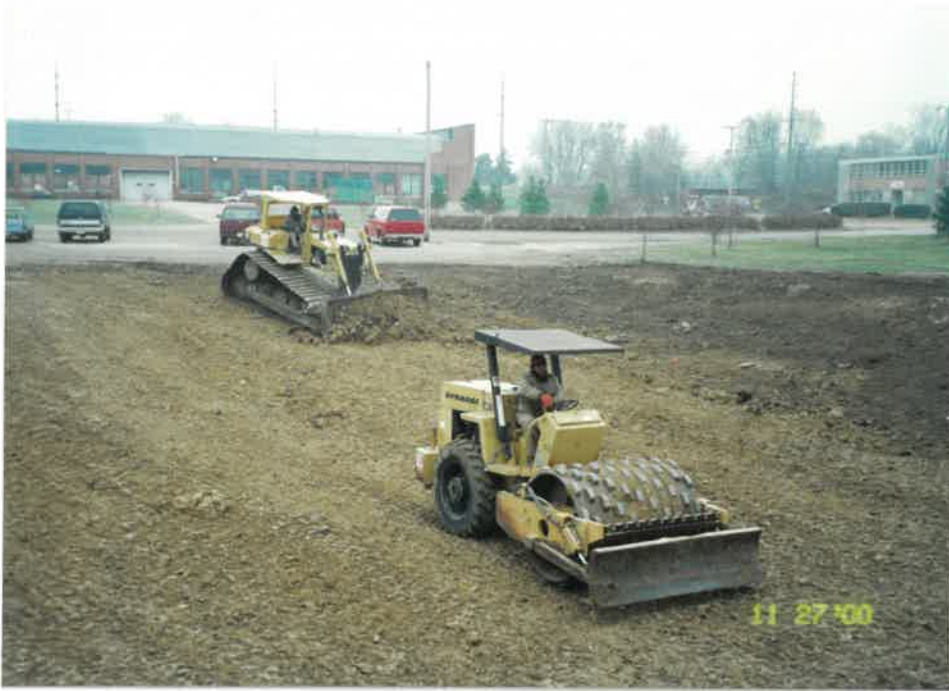
Photograph 1 November 27, 2000 Description: Backfilling and compacting clayey soil cap on Lagoon No. 1A excavation.
